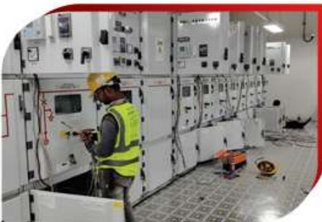
ELECTRICAL POWER UPGRADATION
