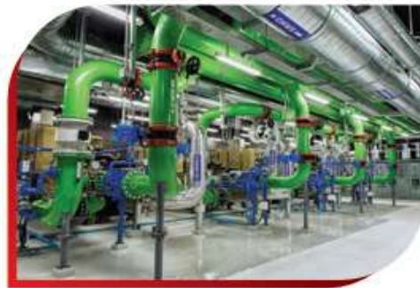
REPLACEMENT & UPGRADATION EQUIPMENT
